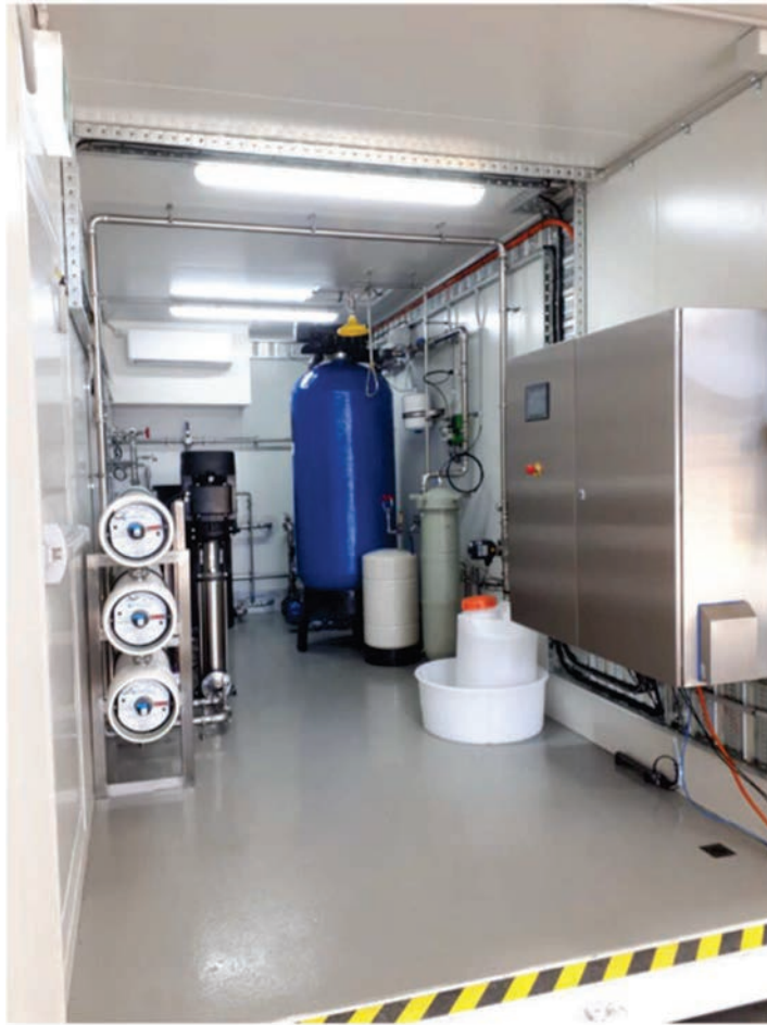
Figure 3: Interior of Reverse Osmosis system.
